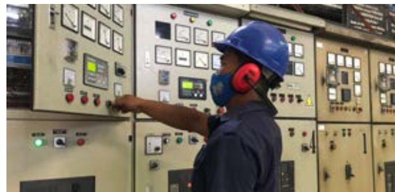
Energy Consumption Monitoring in Begerpang Mill, North Sumatra Pengawasan konsumsi energi di Pabrik Kelapa Sawit Begerpang, Sumatra Utara
